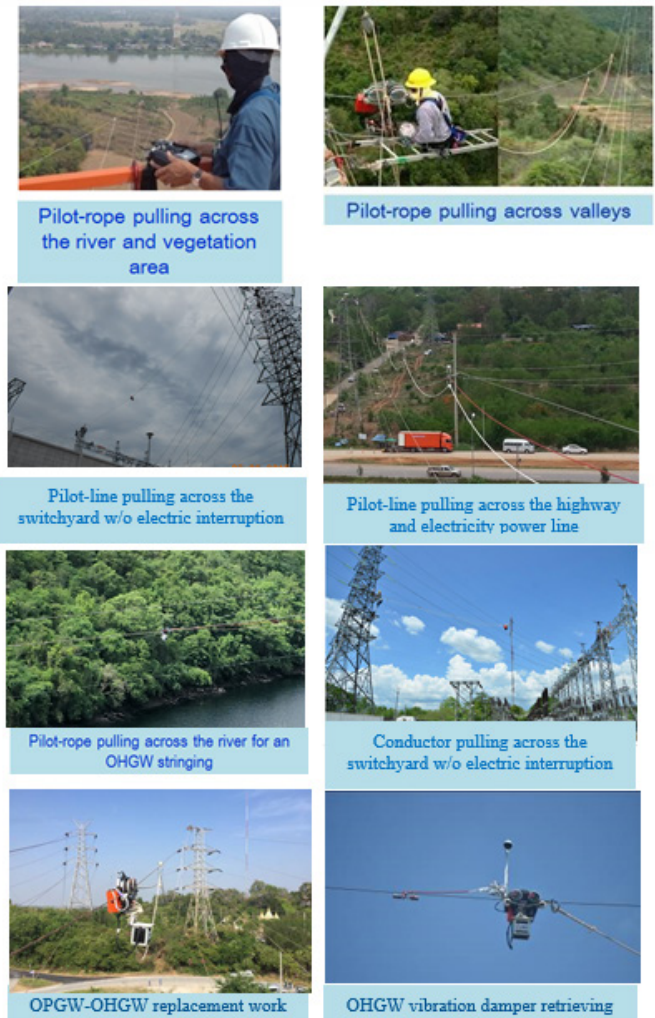
Figure 7: Actual implementations of the transmission line maintenance robot
