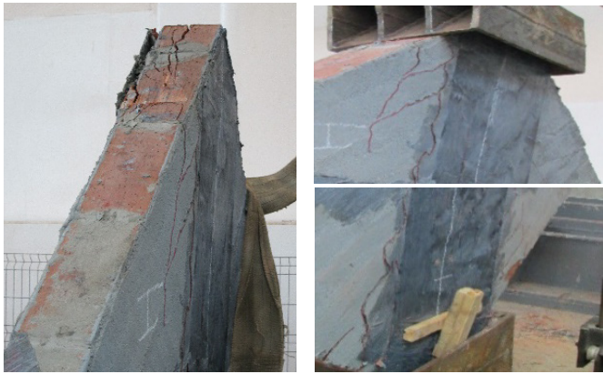
(a) Delamination and shear cracking (Side I)
