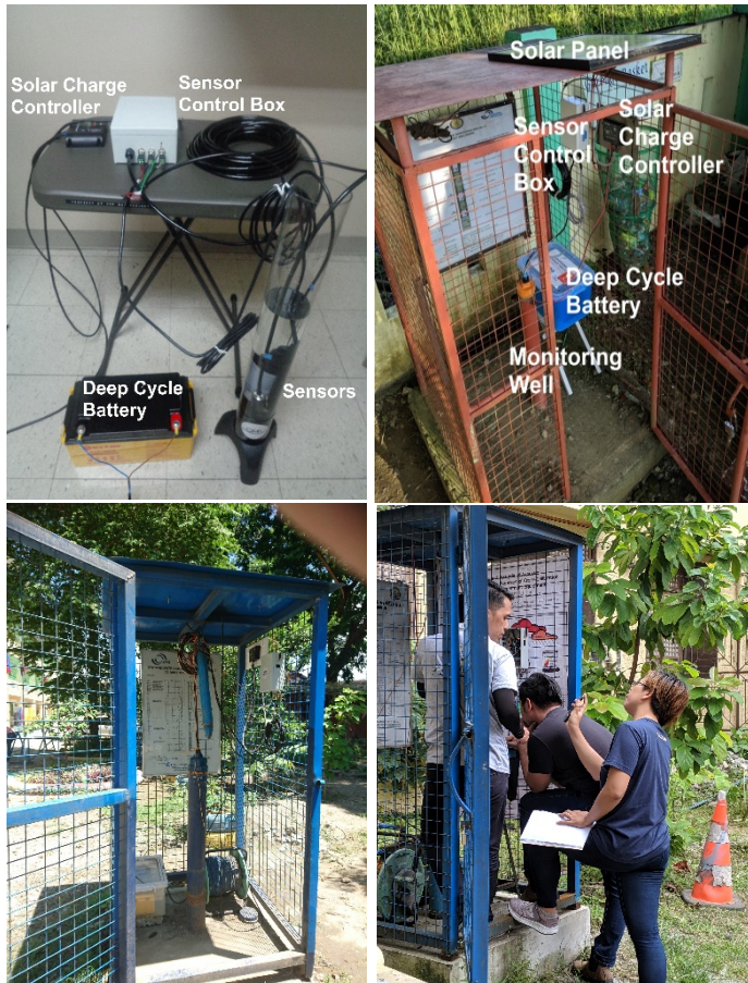
Figure 5: Test setup in a controlled environment (top-left), the setup installed on some of the groundwater monitoring wells (top-right), and the team during one of the system installations (bottom-right)
