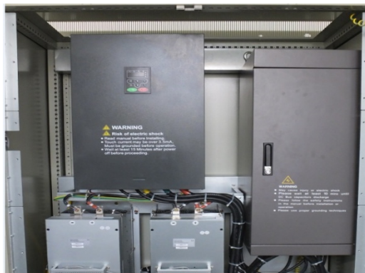
Figure 17. Picture of electric multi-drives equipment.
