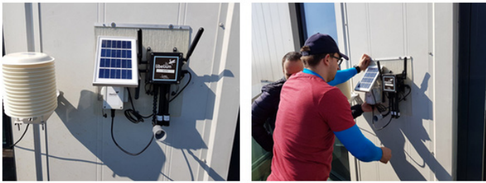
Figure 8: Installation of the measuring equipment Libelium SCP at the CAMPUS center
