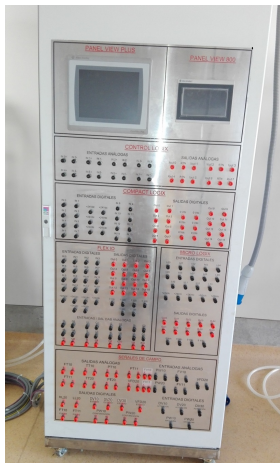
Figure 3: The supervision module
