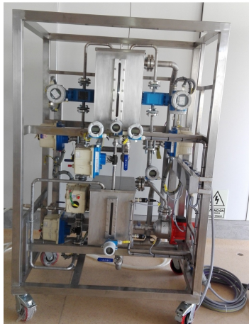
Figure 2: The multipurpose plant
